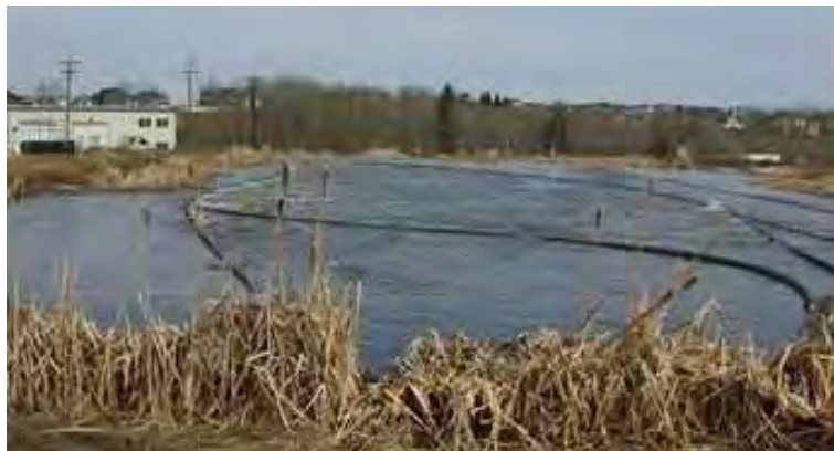
Figure 4-6 Aeration Pipe Laterals in Cell 1
