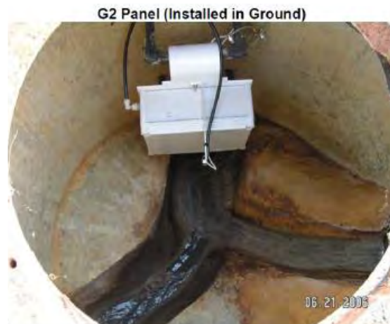
Figure 5-6 In-Pipe Dosing Station in a Manhole
